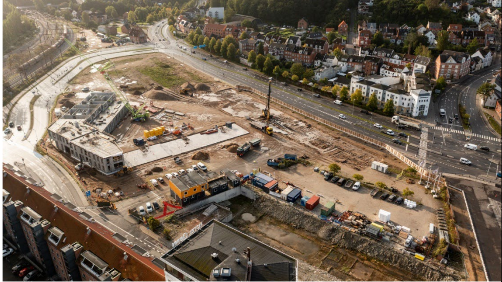
September 2023 – on going construction of residential structure – sold part of project. Pile foundation of S6 (machine) 50% complete.
